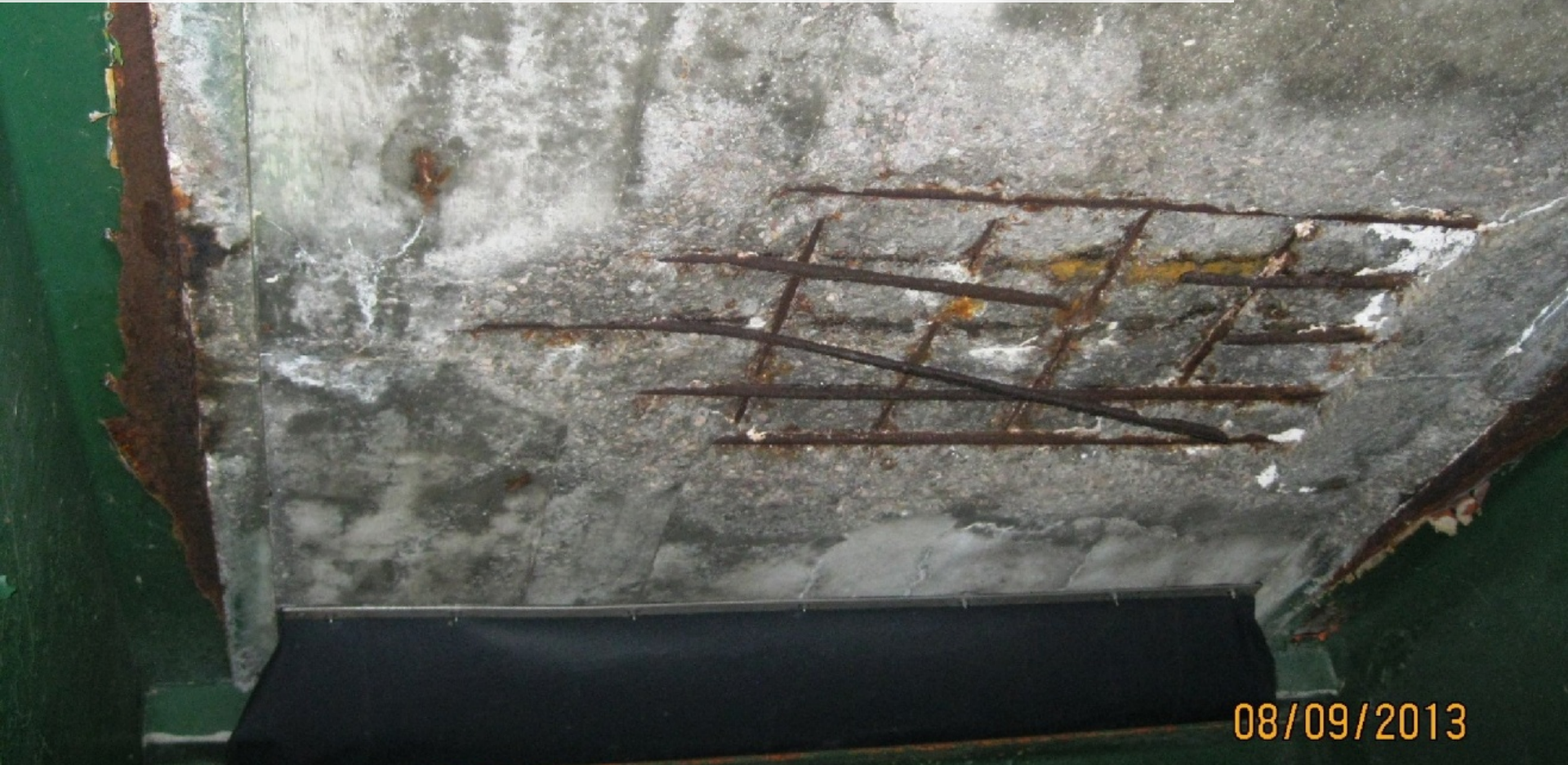
Heavy Deterioration of Deck
